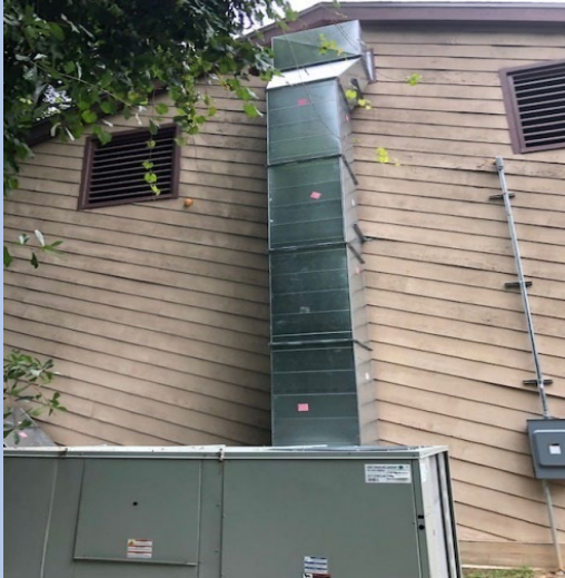
New HVAC unit/duct
