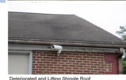
Deteriorated and Lifting Shingle Roof
