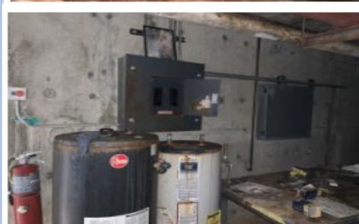
Water Heater and Panels
