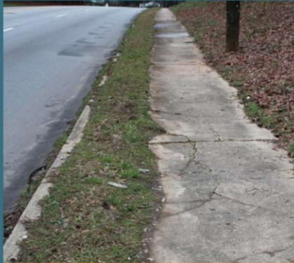
Some cracks in sidewalk
