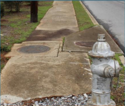
Significant deterioration and/or impediments in sidewalk
